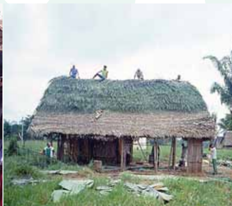
Building a "pahuichi" house in Galilea, in the Cavineño community, Beni River, Bolivia (Photo courtesy of Johannes Stahl)
