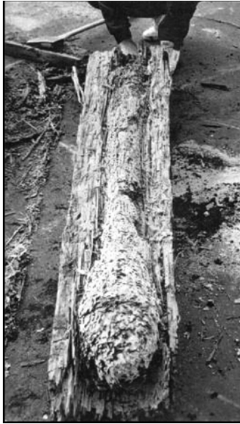
Figure 1. Coptotermes acinaciformis nest found concealed within imported Australian utility pole.
