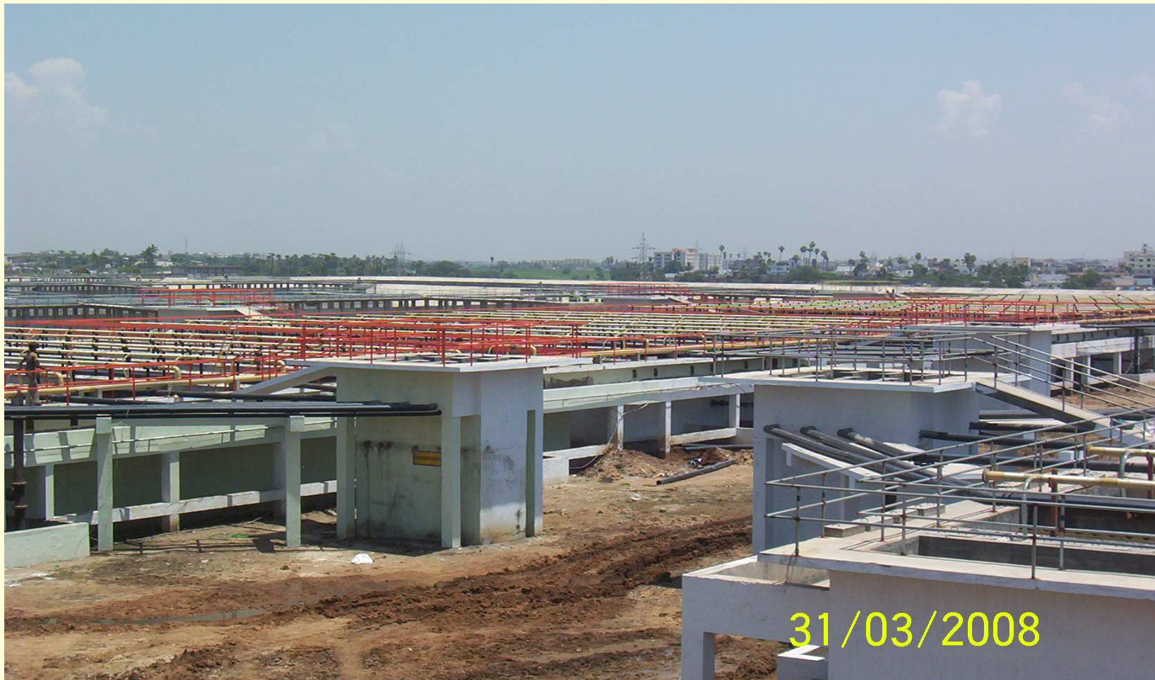
Distribution Box & UASB Reactors
