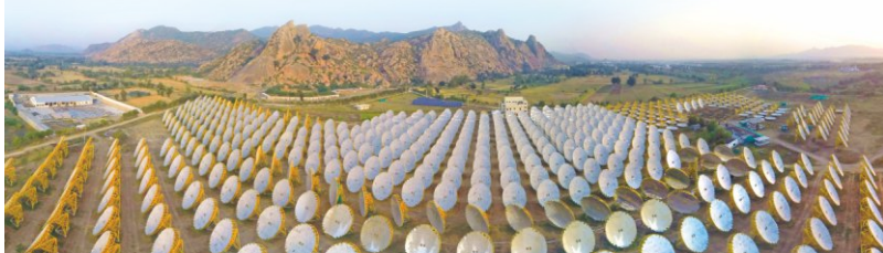
'India One' Solar Thermal Power Plant
