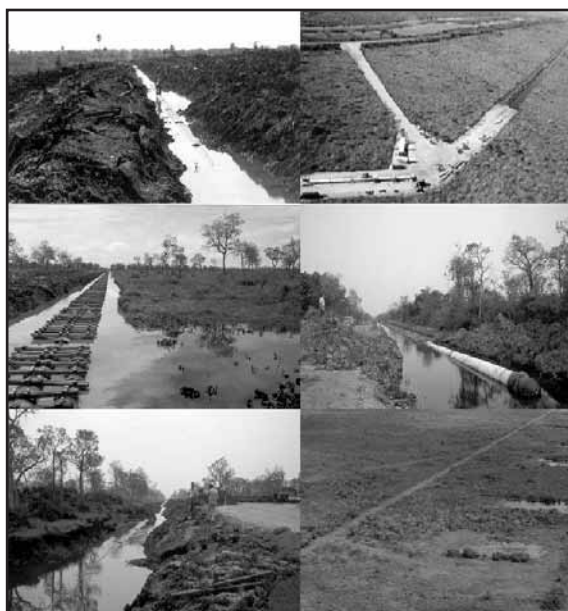
Shown in sequence, from left to right, top to bottom: the excavated trenches, platforms, pipe sections with floaters, pipes placed in trench, flooded trench, and current view of the ROW in the Pantanal.
