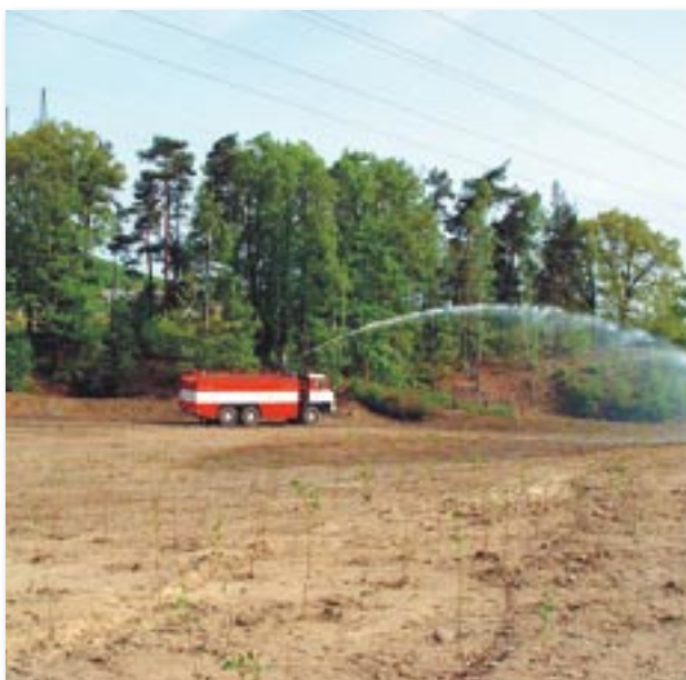
• Process of dumpsite reconstruction in the village Kozly
